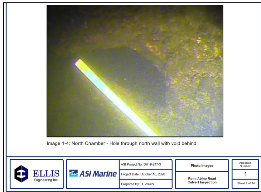
Figure 30 Underwater inspection defect North wall
